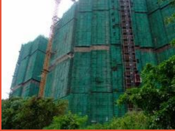
Construction Safety Net
