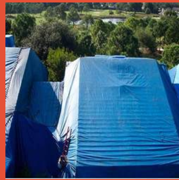
Stack Fumigation Service
